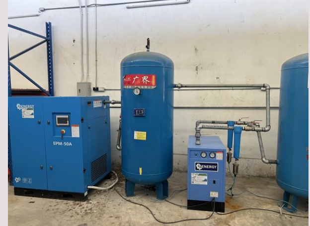
Air Compressor Plant
